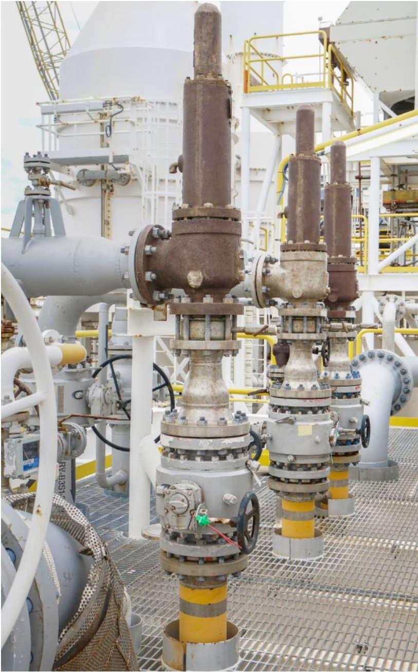
Figure 2. Example of pressure relief valves located together on platform
